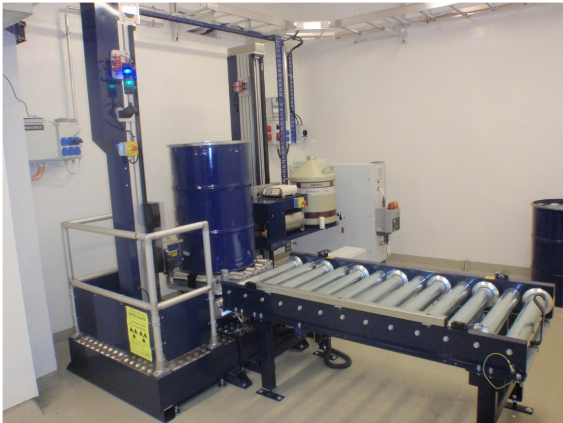
Figure 1. WR-SGS installed in the waste measurement room at Loviisa Nuclear Power Plant
